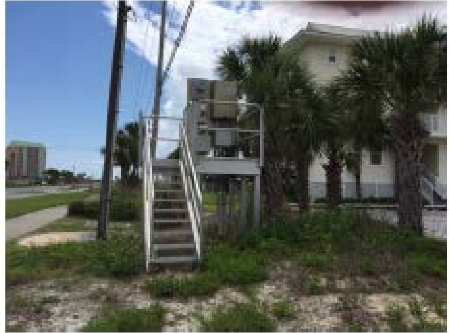
Elevate electrical panel
