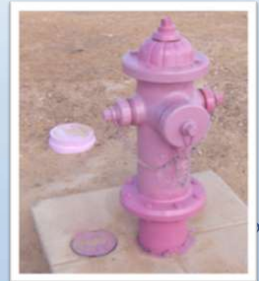
Reclaimed Water Fire Hydrant
